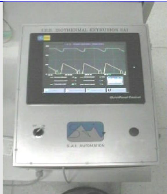
Fig. 2: Central control panel
