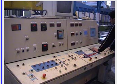
Fig. 9) Central Control Board
